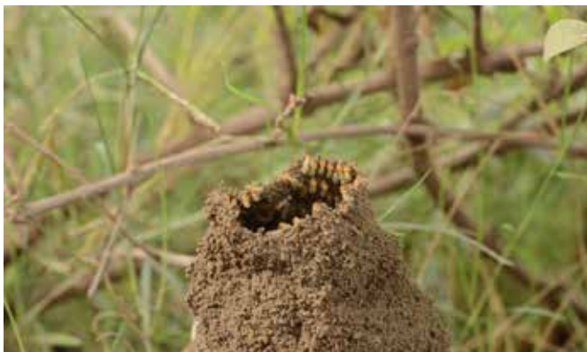
These mud deposits indicate active termites
